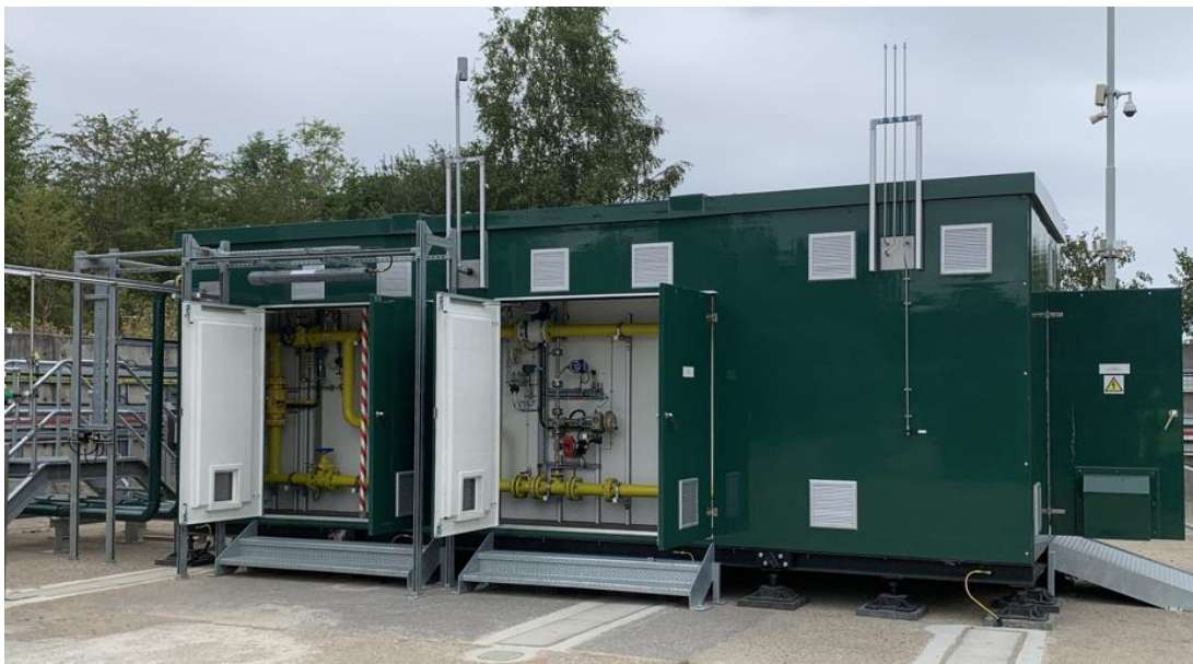
Figure 1, the purpose designed and built blending unit
