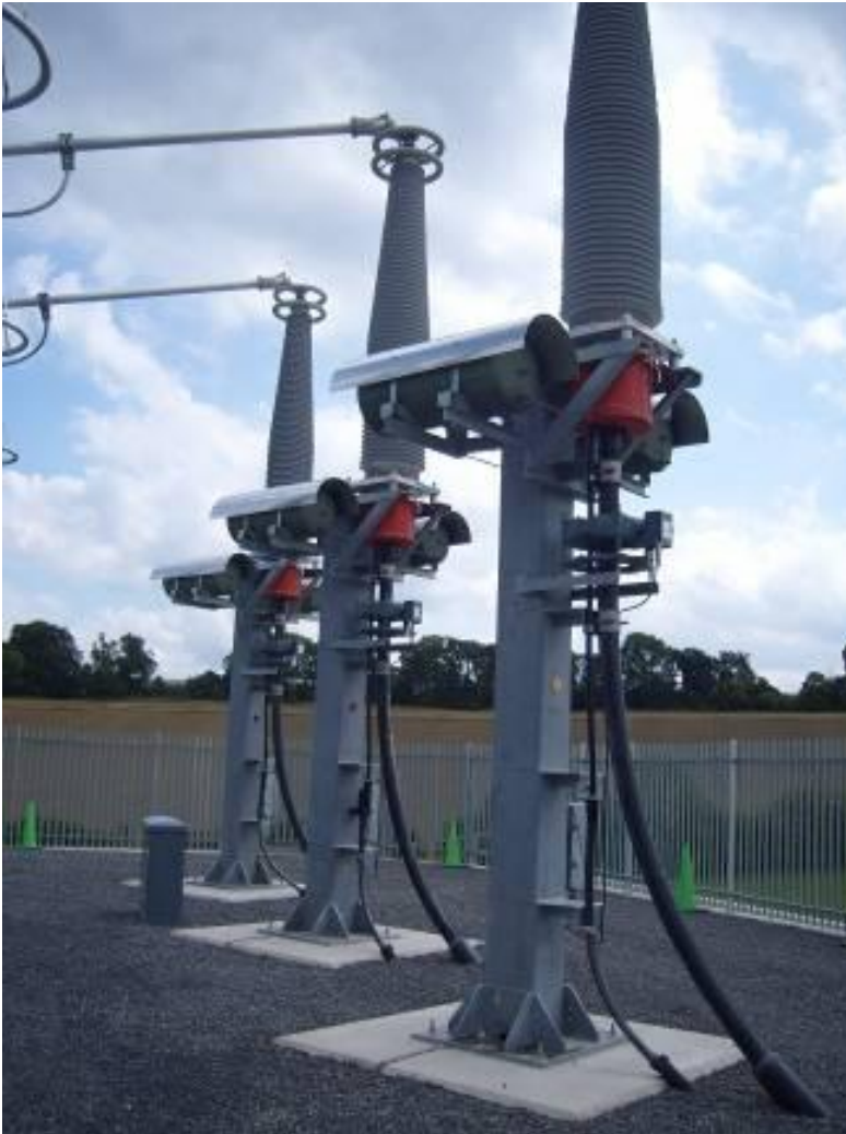
Figure 22 – 400kV terminations installed near Goring
