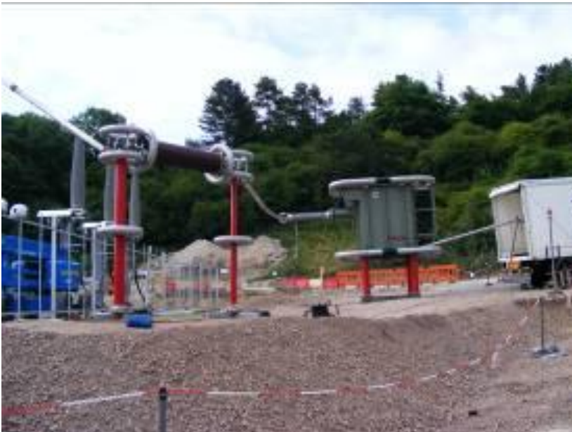
Figure 26 – Cable AC test voltage equipment
