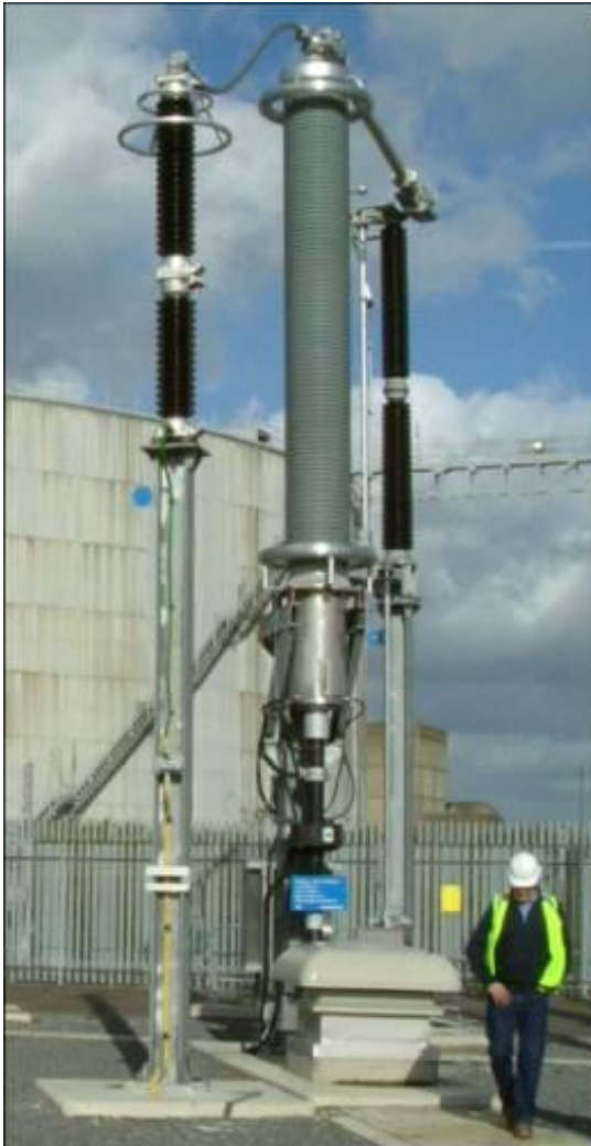
Figure 21 – 400kV cable outdoor sealing end (ODSE) termination
