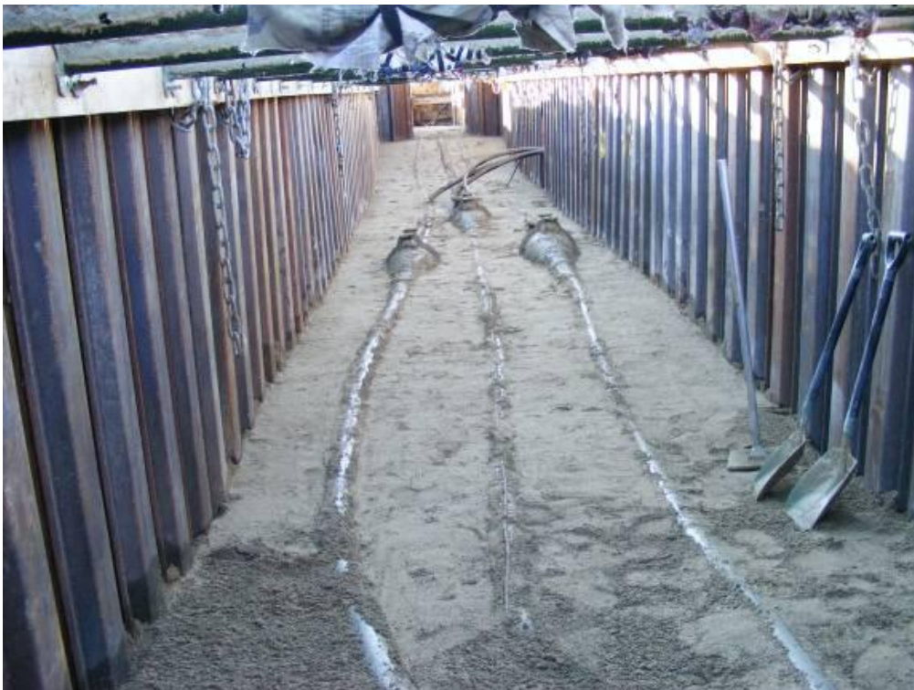
Figure 19 – EHV joint bay containing three Joints
