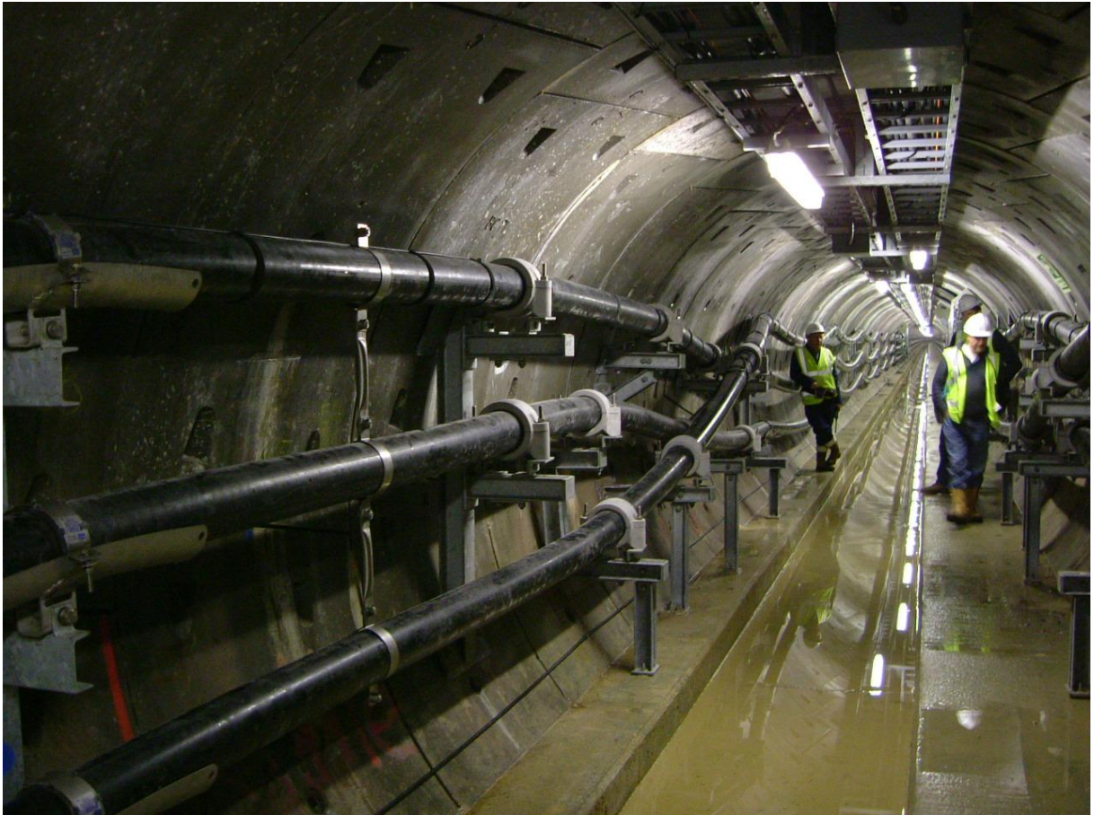
Figure 3 – 400kV cable tunnel crossing beneath the Thames at Dartford
