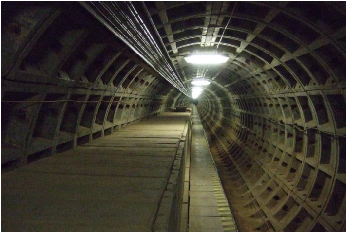
Figure 45 – Wimbledon–New Cross cable tunnel
