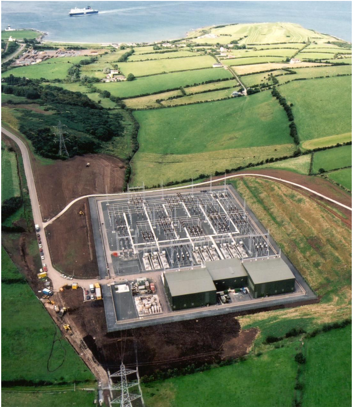
Figure 5 – Ballycronan More 500MW CSC converter station
