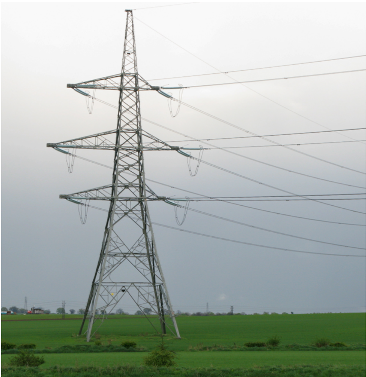
Figure 2 – L6 D60 tower with 400kV insulators and twin conductor bundle
