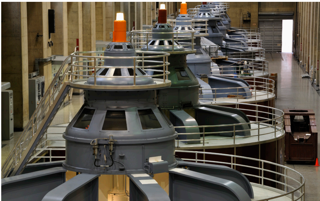
Large Hydro Electric Power Plant Generators
